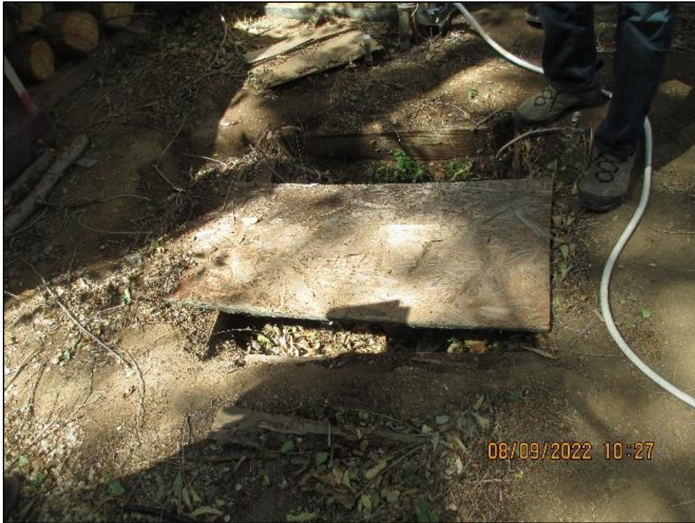
Image 4: Unsecure plywood cover placed above West Cesspool.
