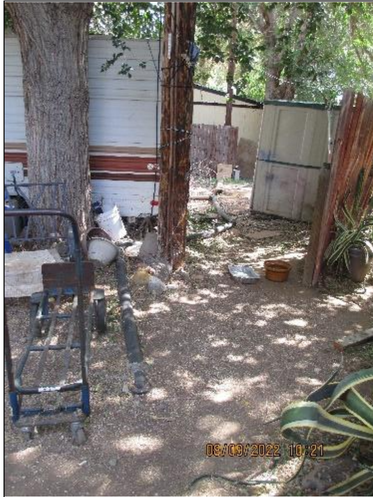
Image 3: Black above-surface pipeline between two mobile homes on the southwest side of the Park.
