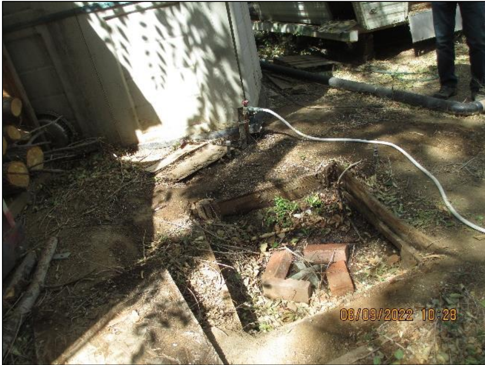
Image 6: Another angle of West Cesspool. white hose, and potable water line as pictured/referenced in Image 5.
