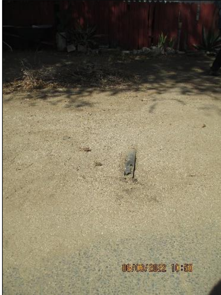
Image 13: Open black pipe protruding from ground. Appeared to connect to black pipes in Image 12.
