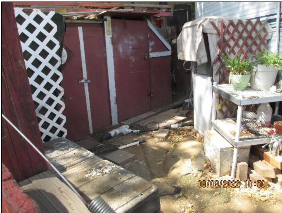
Image 12: Black pipes connected to washer and dryer and branches off behind the mobile home. Appeared to connect to the pipe pictured in Image 13.
