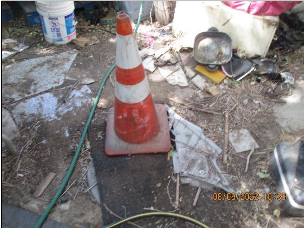
Image 9: East Cesspool was located under traffic cone and black house mat. Green hose connected to potable water faucet pictured on the left.
